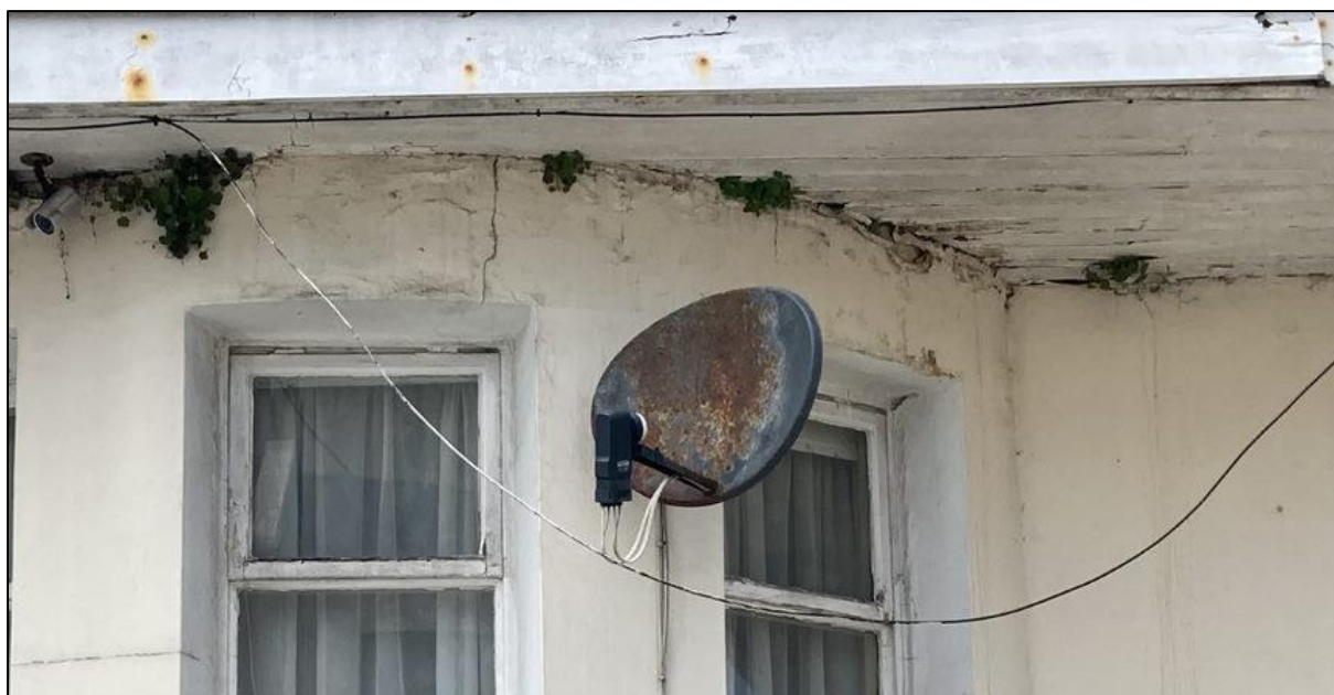
Figure 3-8: An example of a loose wire from AECOM inspection surveys
