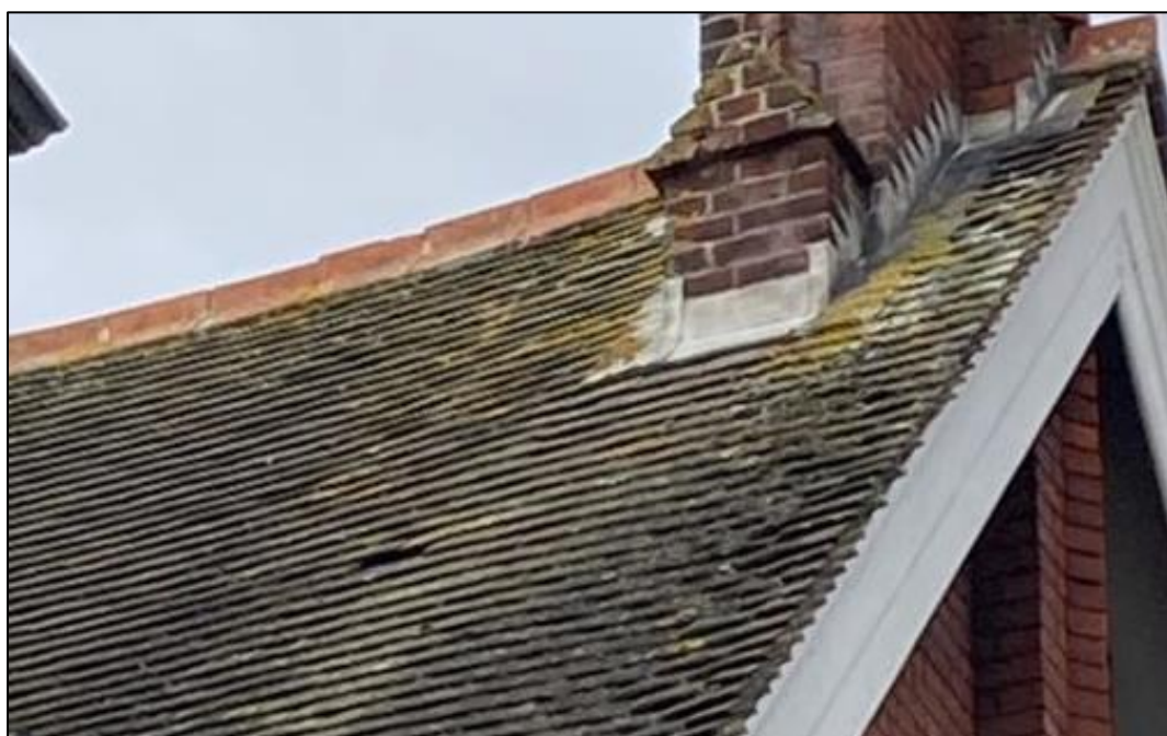
Figure 3-1: An example of loose roof tiles and moss from AECOM inspection surveys
