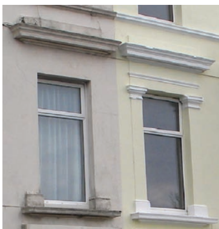
Picture 48 Loss of plaster details, Upperton Gardens.
