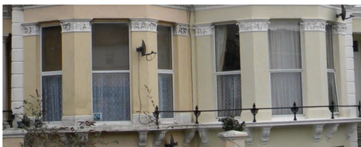
Picture 39 Missing sections of cast-iron sill guards.
