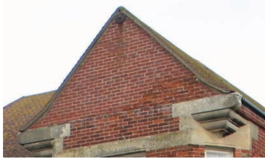
Picture 16 Skew corbels to no. 56 Upperton Gardens.
