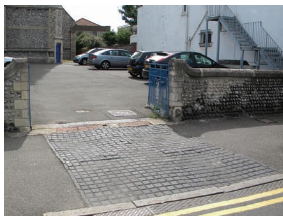
Picture 48 Staffordshire Blue bricks to Christ Church crossover, Seaside.
