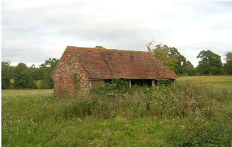
Poor condition of barn along Church Lane
