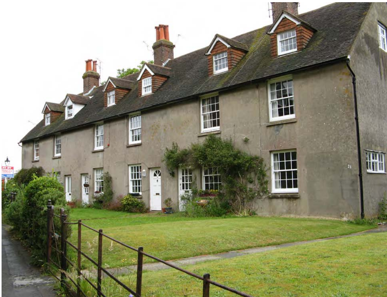
An Article 4 Direction could help preserve the character of this building in The Twitten
